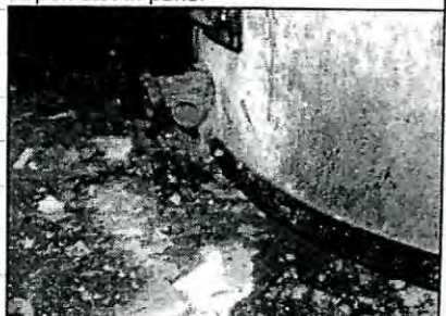
Leak at water heater
