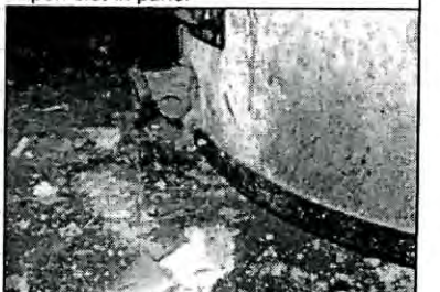
Leak at water heater
