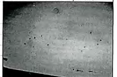
Wood boring beetle damage
