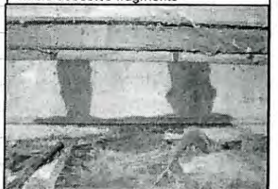
Water intrusion, west under gym
