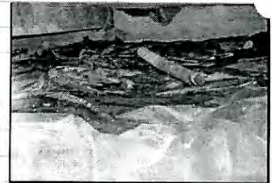
Standing water, NW under gym
