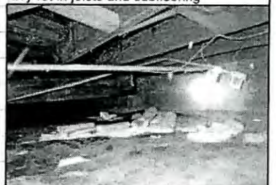
Friable asbestos fragments
