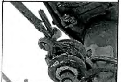
Bare wires on service drop conductors
