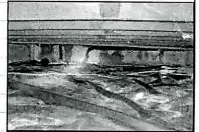
Water intrusion, W end, loose wiring.
