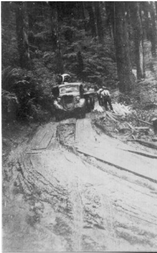
Planking the road at Frog Creek, a few hundred yards above the top of Golden Falls.
