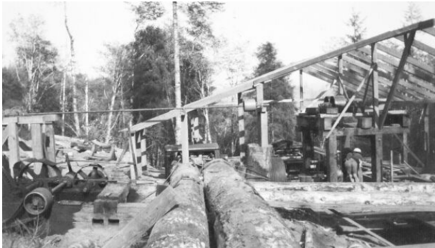
Hollow Stump mill under construction, 1945. Drag saw, left, log rollway, right. Roof is unfinished.
