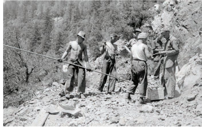
Blasting crew from Camp Rand preparing a shot near the Graves Creek Bridge, 35 miles above camp Agness, ca. 1935. On many occasions, the truck roads involved a lot of hand labor by the CCC men on the road crews. Photo courtesy of the U.S. Forest Service Ranger Station at Gold Beach, Oregon.
